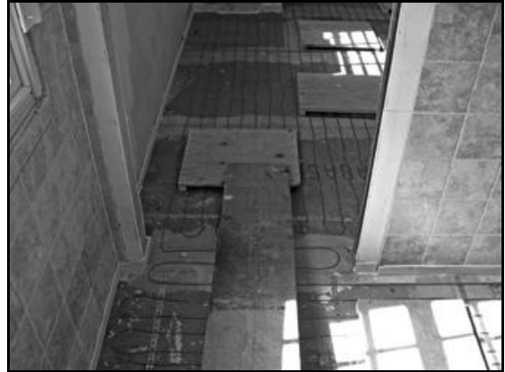
Figure 1: Create a walkway over the unprotected heating cables.
