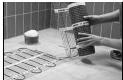
Figure 5: Cut mesh backing to turn the heating mat for the desired layout.
